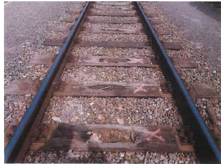
Marked sleepers which can't be treated
